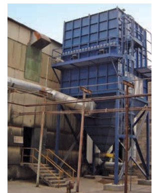
324MBWS10 Shingle Manufacturing
