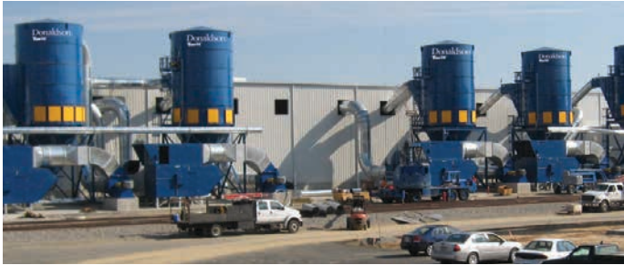
776RF at Wood Furniture Plant
