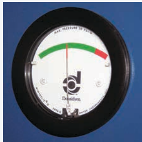
Differential pressure gauge(s) identifies filter maintenance.
